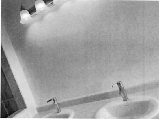
148266 - 1 - MIRROR~MIRROR NOT INSTALLED THROUGHOUT
