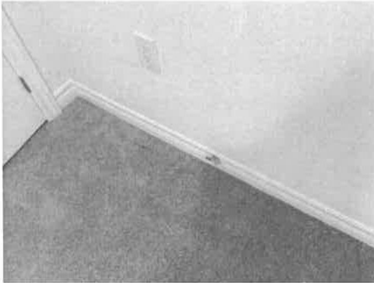
151427 - 1 - NOTE:~DOOR STOPPER NOT INSTALLED
