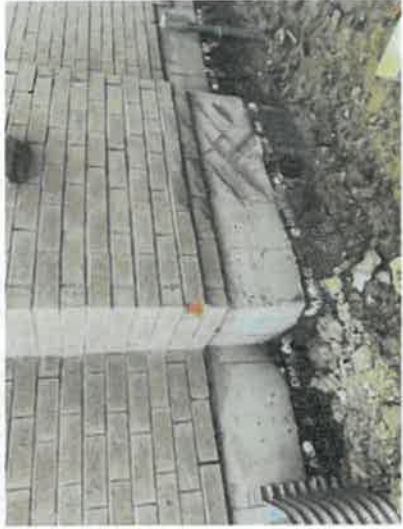
EXTERIOR LEFT SIDE OF HOUSE 4) LARGE CHIPPED BRICK LEFT SIDE OF HOUSE LEFT OF FIREPLACE 5) INSPECT CHIPS ON BRICKS ON RIGHT SIDE OF HOUSE.
