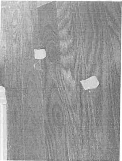
151351 - 1 - FLOORING~LARGE CHIP ON 4, 6 PLANK INFRONT OF MAIN BATH
