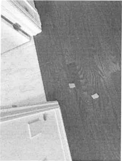
151351 - 2 - FLOORING~LARGE CHIP ON 4, 6 PLANK INFRONT OF MAIN BATH
