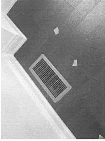
152565 - 1 - FLOORING~TWO SCRATCHES ON HARDWOOD IN FRONT OF AIR RETURN RIGHT OF STAIRS
