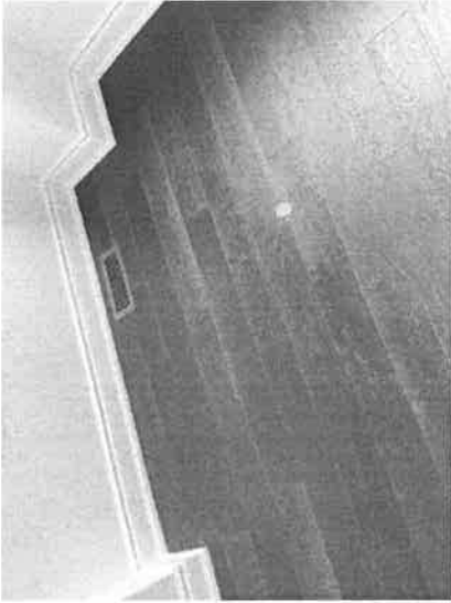
152558 - 1 - FLOORING~CHIP ON SIX HARDWOOD PLANK FROM RIGHT HEAT REGISTER RIGHT OF FIRE
