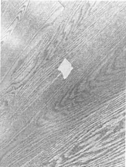
149397 - 1 - FLOORING~CHIP ON 9TH PLANK FROM LEFT WALL AT ELECTRICAL OUTLET
