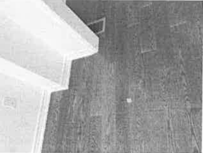
149397 - 2 - FLOORING~CHIP ON 9TH PLANK FROM LEFT WALL AT ELECTRICAL OUTLET
