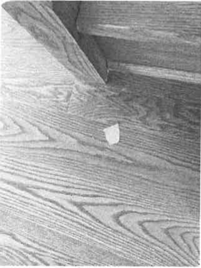
149402 - 1 - FLOORING~CHIP ON 2ND HARDWOOD PLANK INFRONT OF STAIRS TOO 2ND FLOOR
