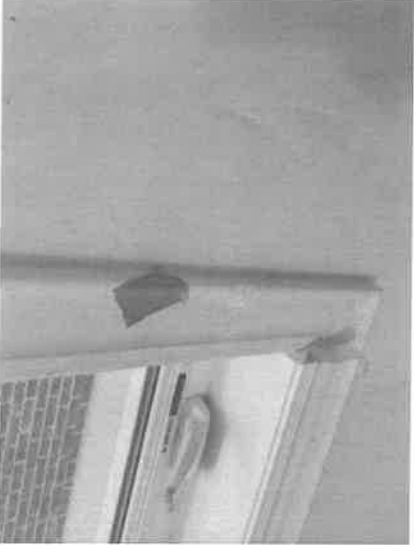
168019 - 1 - TRIM~REPLACE WINDOW TRIM DAMAGED
