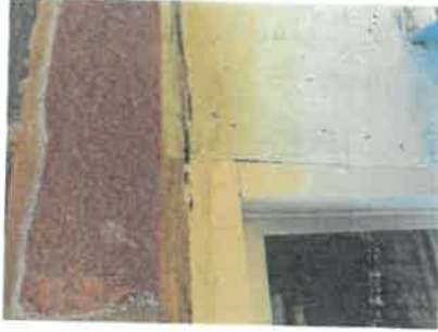
178121 - 6 - 20240804_124901_resized - svc to fix caulking - see photos for locations - BOOKED FOR AUG 19
