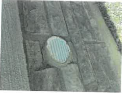
178121 - 1 - 20240804_124830_resized - svc to fix caulking - see photos for locations - BOOKED FOR AUG 19
