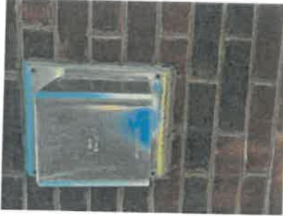
178121 - 4 - 20240804_124915_resized - svc to fix caulking - see photos for locations - BOOKED FOR AUG 19
