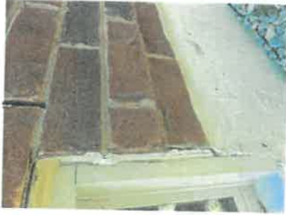
178121 - 5 - 20240804_124852_resized - svc to fix caulking - see photos for locations - BOOKED FOR AUG 19
