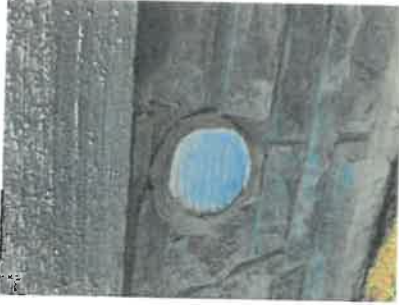
178121 - 2 - 20240804_124832_resized - svc to fix caulking - see photos for locations - BOOKED FOR AUG 19
