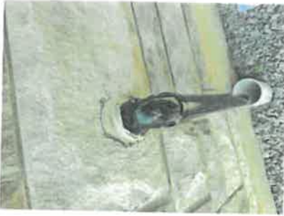
178121 - 3 - 20240804_124836_resized - svc to fix caulking - see photos for locations - BOOKED FOR AUG 19
